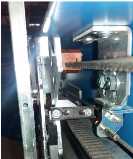
Pic 8: Stud/contact bridge at the unlocking device
